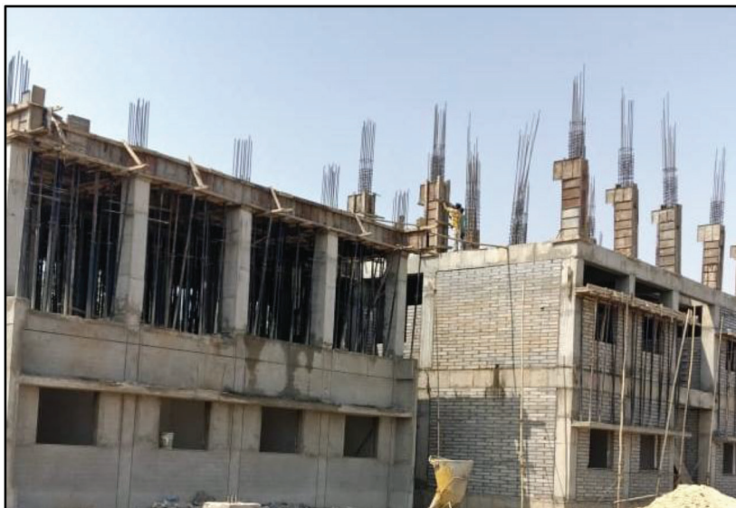
Slab & Column, Reinforcement and RCC work in progress at Administration Building of Bridge Workshop, Ahmedabad, Gujarat
