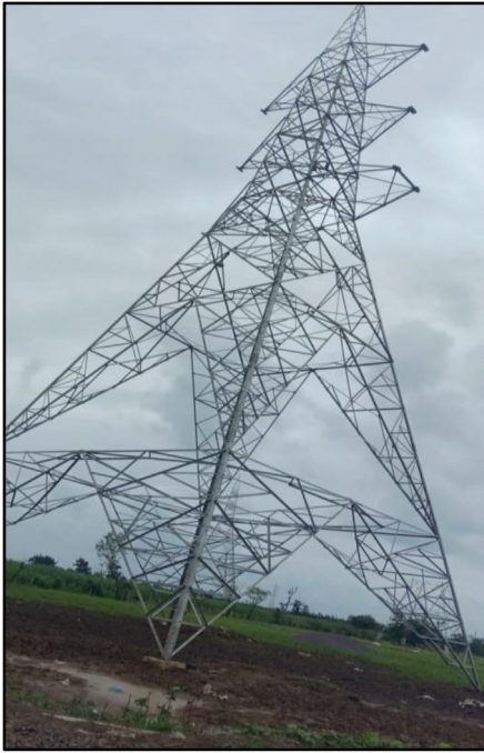
Tower erection of 220 kV line (i.e. Vapi / Kharadpade & Vapi / Mangalwada Crossing chainage 169.334), Vapi, Gujarat
