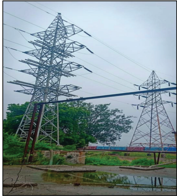
Tower erection and Stringing work by Torrent Power Limited at Vatva, Ahmedabad, Gujarat
