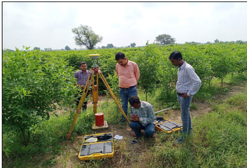
Right of Way Marking and Pillar Fixing at Kothi Vantarsha Village, Bharuch District, Gujarat
