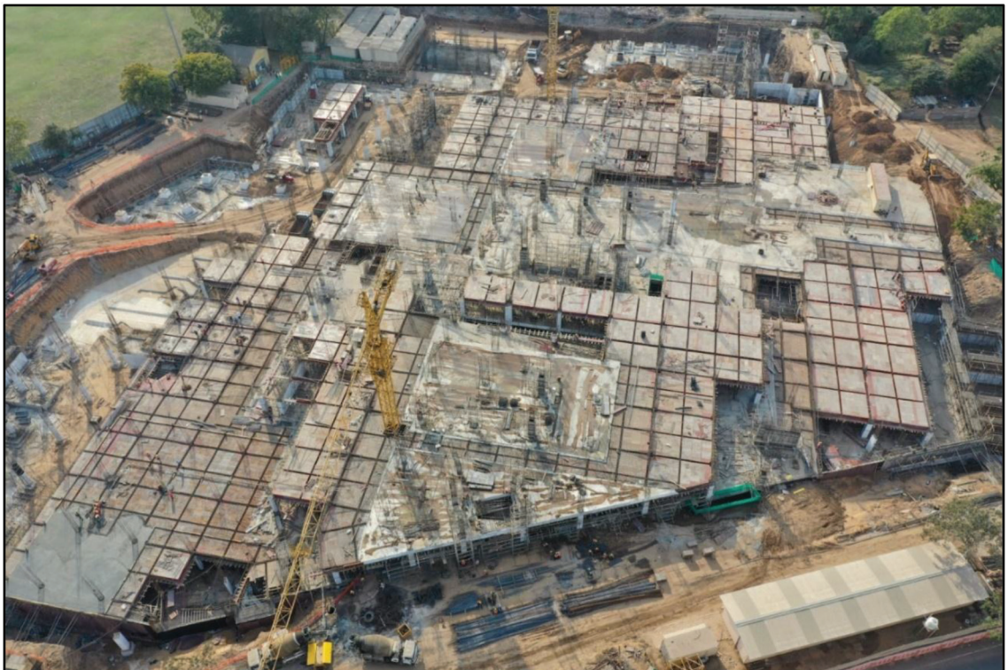
Construction of Ground Floor Slab in progress at Passenger Terminal Hub, Sabarmati, Gujarat
