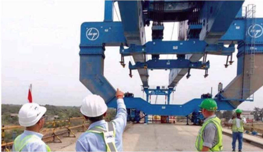
NHSRCL MD Satish Agnihotri explaining to Japan Ambassador Satoshi Suzuki about the state of the art technology, techniques, equipment and machinery at use for expediting the civil work for Bullet Train project
