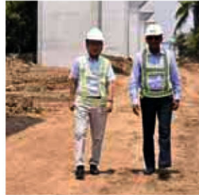
NHSRCL MD S Agnihotri and Japanese Ambassador to India Satoshi Suzuki at a joint inspection of the Bullet Train at the construction site in Navsari and Surat in Gujarat.
