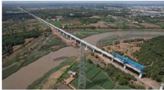
Picking up pace: The Purna river bridge is the second of the bridges to be completed as part of the project. SPECIAL ARRANGEMENT
