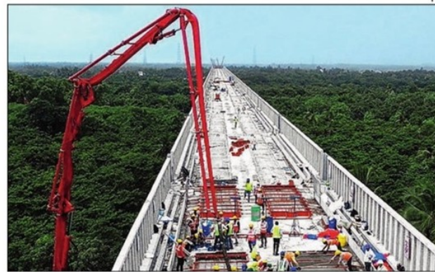
It is for the first time that the J-slab ballastless track system, a feature of Japan's high-speed rail system Shinkansen, is being used in India
