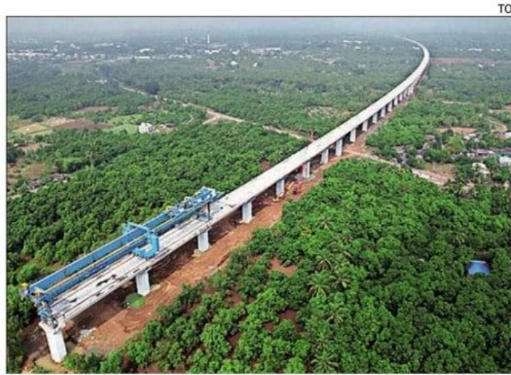
HSR stations at Vapi, Bilimora, Surat, Bharuch, Anand, Vadodara, Ahmedabad and Sabarmati in Gujarat are at various stages of construction
