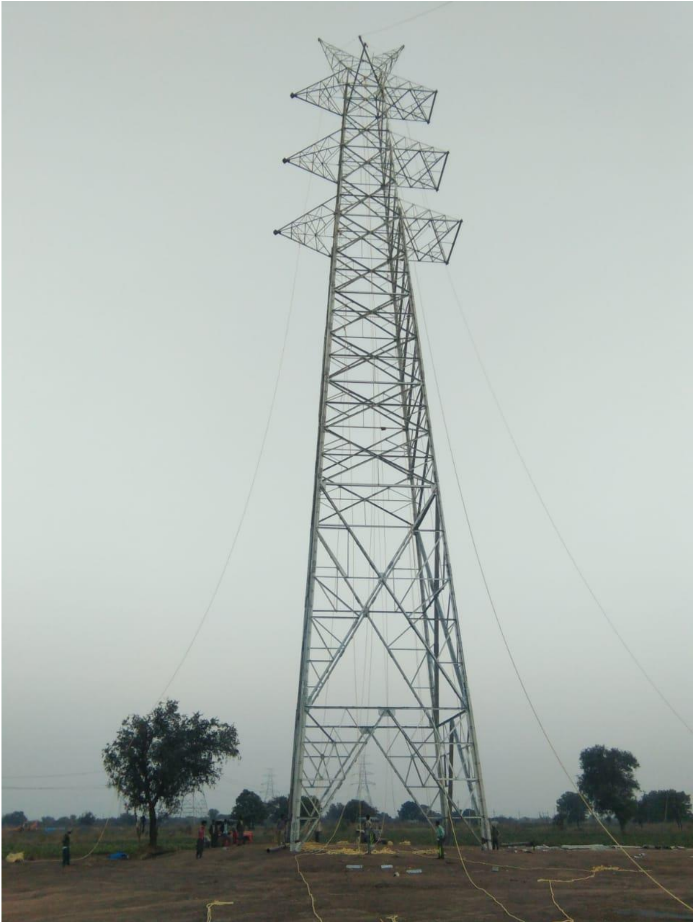
Images: Relocation work of 66 kV extra high tension line in Surat area
